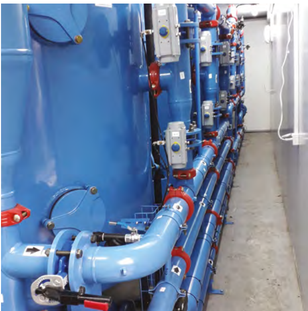
REINO UNIDO | BLÜCHER SPECIALISED MEDIA PRESSURISED FILTRATION SYSTEM
